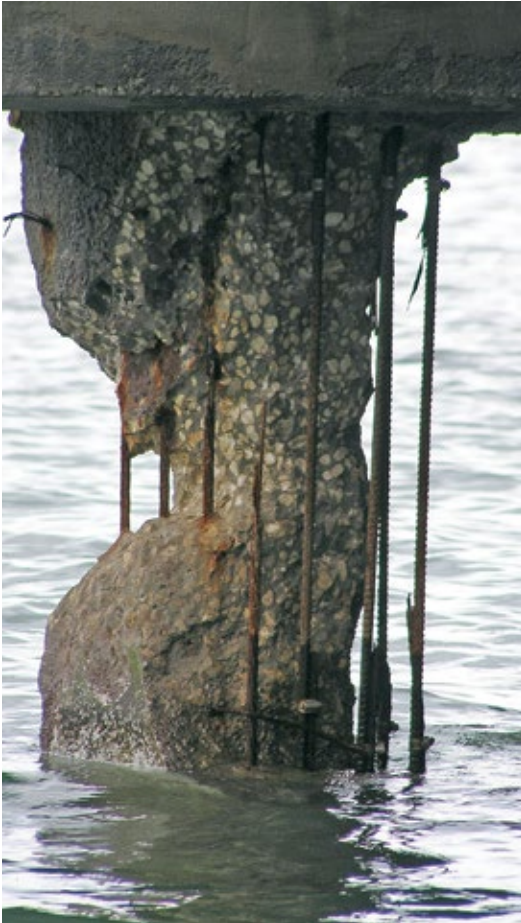
Corrosion of Prestressed Concrete Pile in Saltwater Tidal Zone
