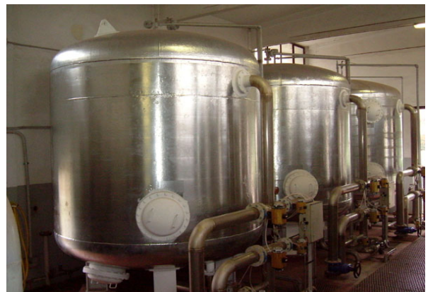
Condition of Tanks after ZincTape Application
