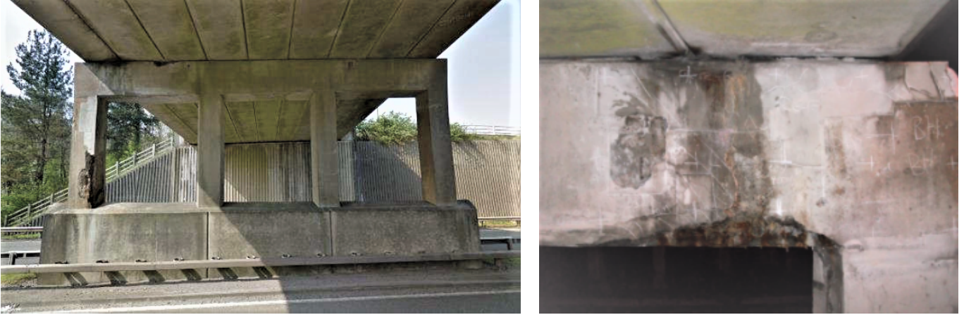
Figure 4 Part of Pier-2 in the bridge in South Wales showing the Abutment in the background (left) and typical damage of the structure from chloride-induced corrosion of the steel reinforcement (right)
