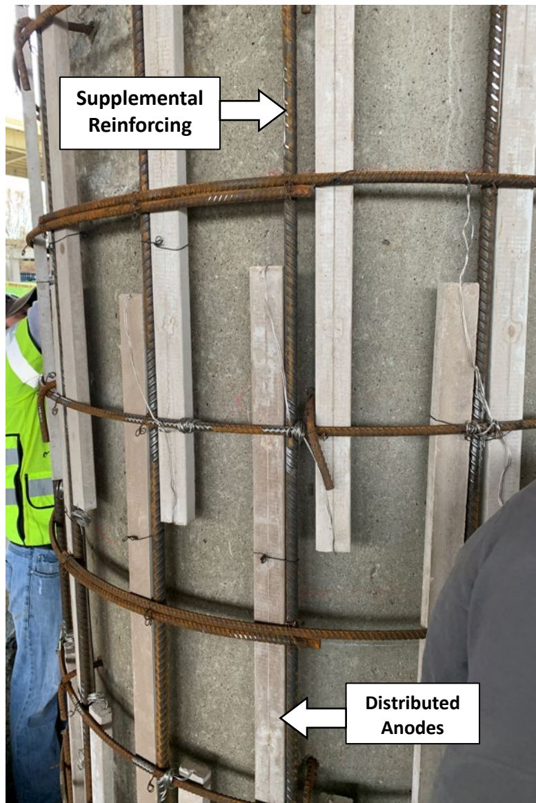
Figure 3: Galvanic Encasement of Heavily Reinforced Column with Distributed Anodes and Supplemental Reinforcing Prior to Concrete Placement, Louisville, KY
