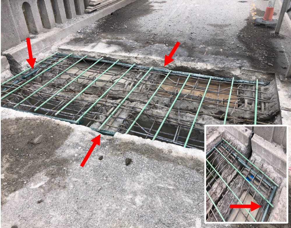
Figure 1: Distributed Anodes in Joint Elimination, McLean County, KY
