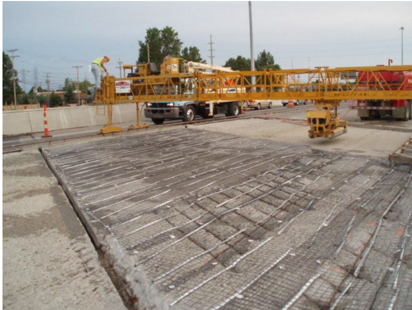
Figure 4: Distributed Galvanic Anodes Incorporated into Bridge Deck Overlay, Cuyahoga County, OH
