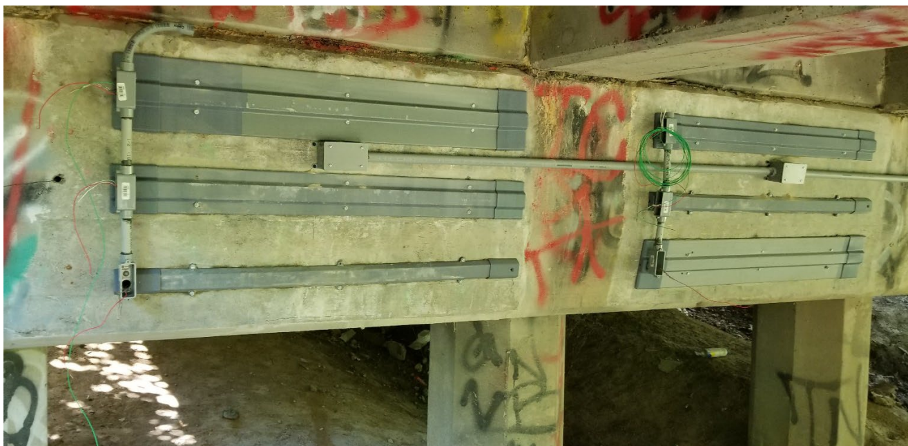
Figure 12: Surface Mounted Distributed Anode Field Study, Louisville, KY
