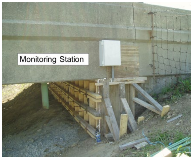
Figure 7: Distributed Anode System Monitoring Cabinet
