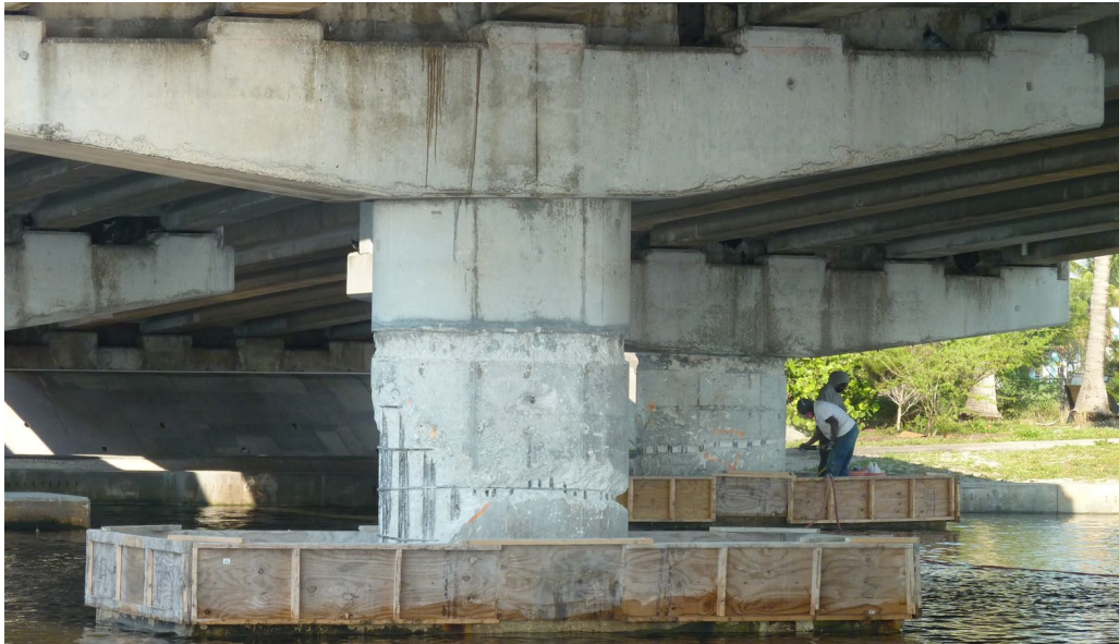
Figure 8: Concrete Damage Revealed After Removal of Structural Steel Jackets
