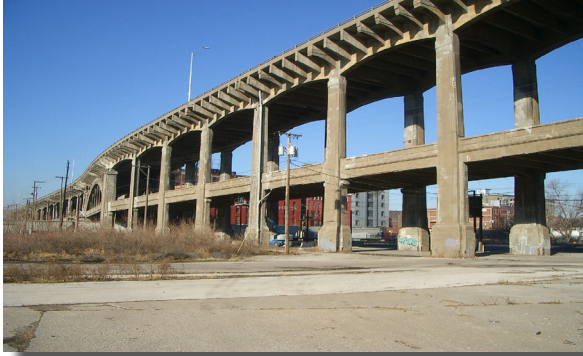
City of Kansas City, MO 12th Street Viaduct, a unique double decked bridge built in the early 1900's
