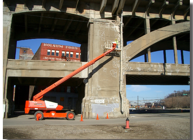
Delamination survey being conducted to identify areas that will need concrete repairs on pier
