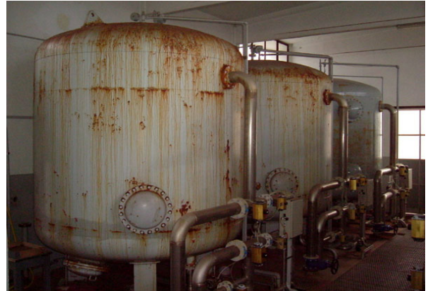
Condition of Tanks before ZincTape Application
