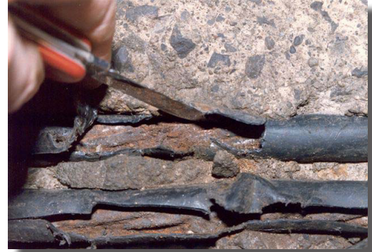
Corroded Cable Within Sheath
