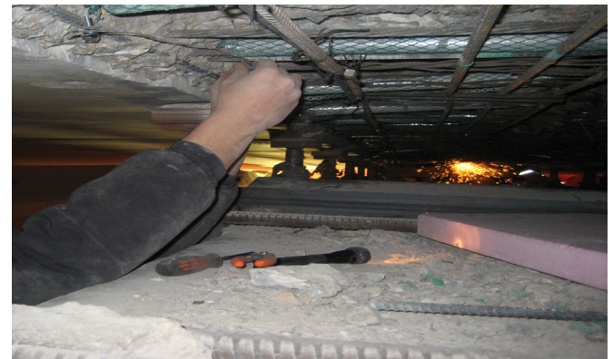
Galvanode DAS anodes installed within bearing area of box girders for corrosion mitigation of embedded steel
