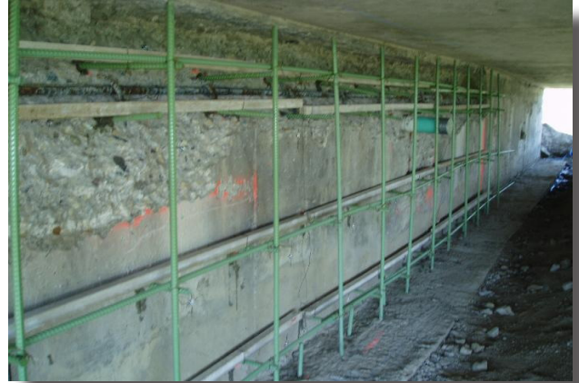
Galvanic anode system on bridge abutment prior to encasement in reinforced concrete overlay
