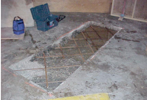
Prepare the area to be repaired in accordance with industry (ICRI) guidelines.
