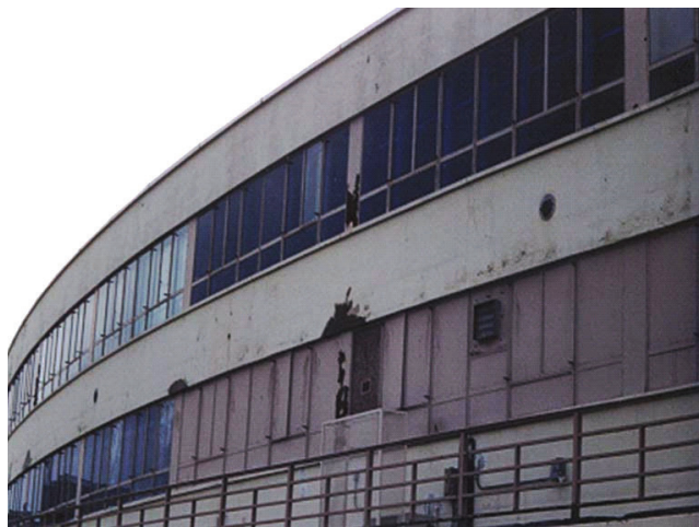
Fig. 3: Deteriorated concrete façade prior to repair
